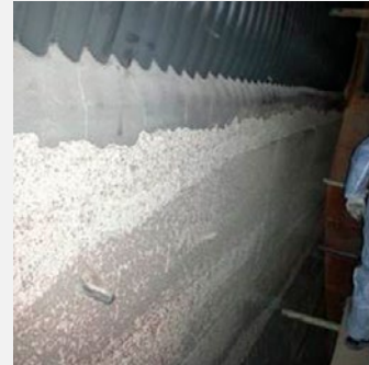
Abrasion in a combustion chamber
