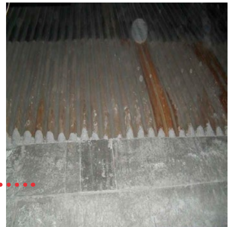
Re-lined lower combustion chamber below free board
