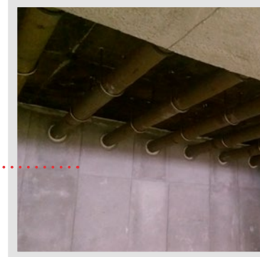
Resistors in the roof of an electrical heating furnace
